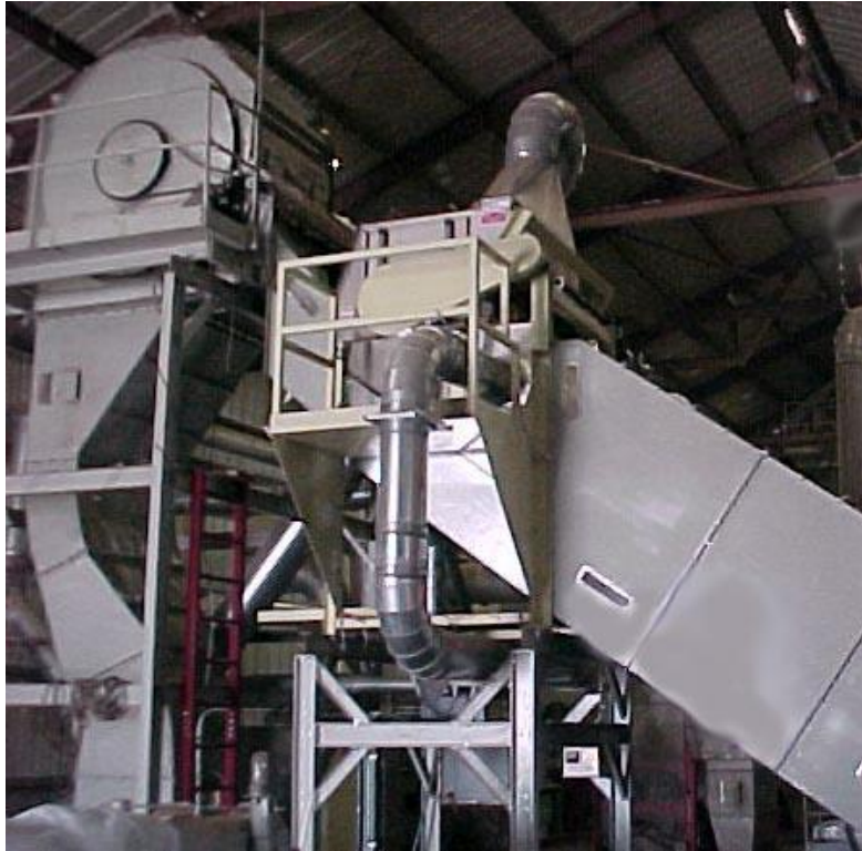
Typical Steamroller Lint Conditioner installation
