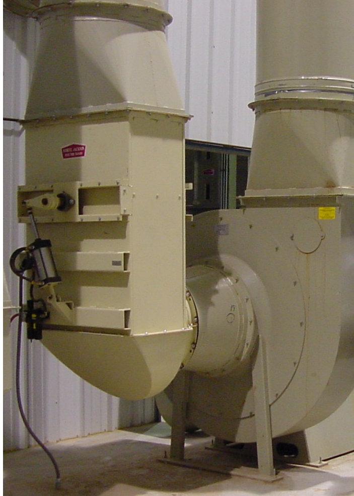
ELECTRIC BANJO installed on first stage inclined cleaner pull fan
