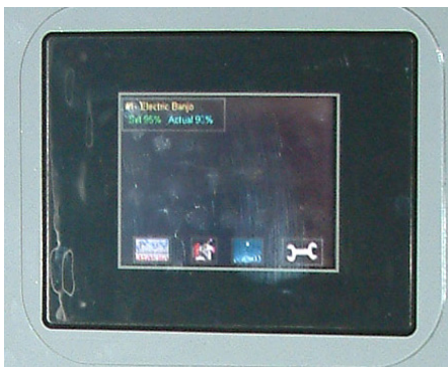
LOCAL PANEL ON CABINET DOOR
