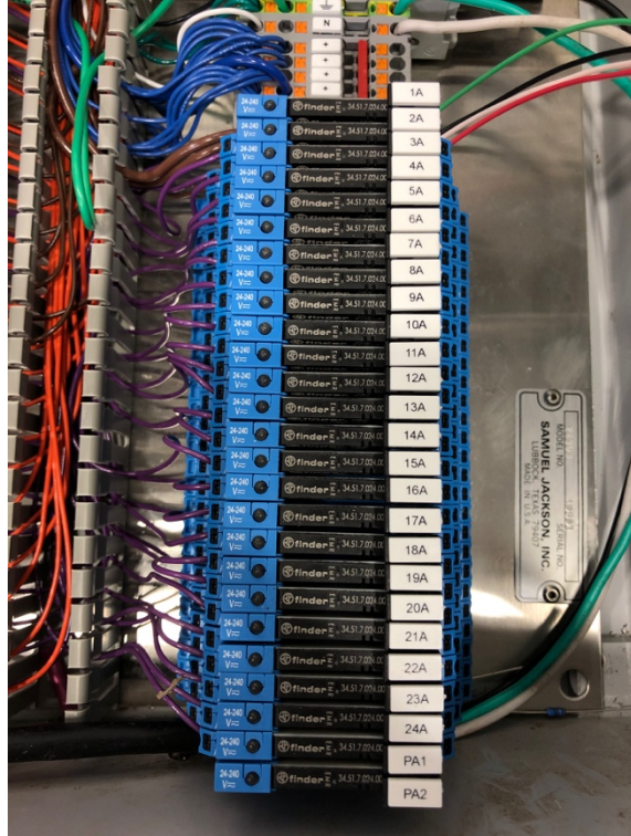
Relay Outputs for Alarms
