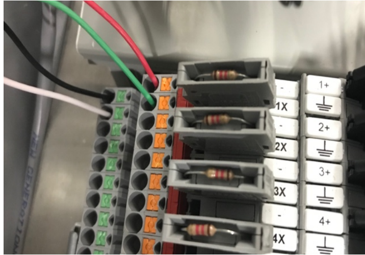
Wiring of Argus on panel
